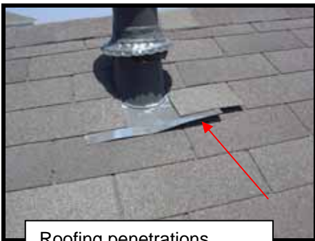
Roofing penetrations should be properly sealed
