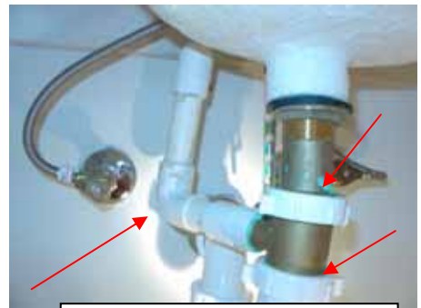
Leak under the sink of the hall bathroom
