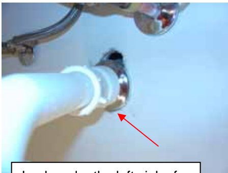
Leak under the left sink of the master bathroom
