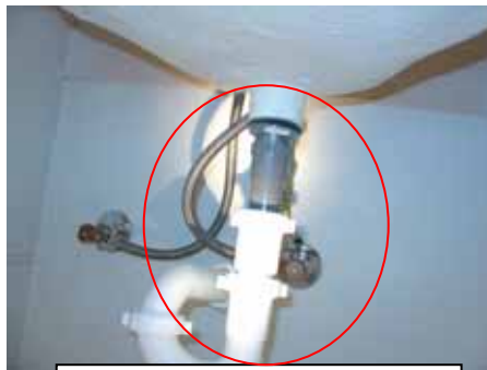
Leak under the right sink of the master bathroom
