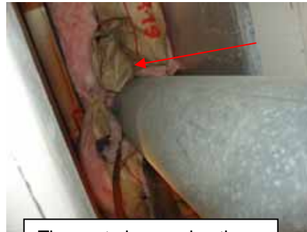
The vent pipe serving the heater does not have safe clearance from combustible materials.
