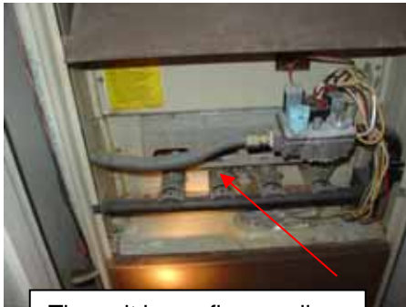
The unit has a flex gas line entering the housing of the heater unit.
