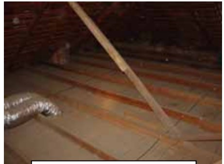
No insulation in attic
