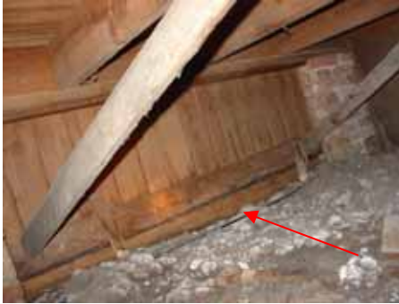
Wood/soil contact in crawl space
