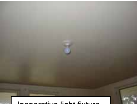
Inoperative light fixture
