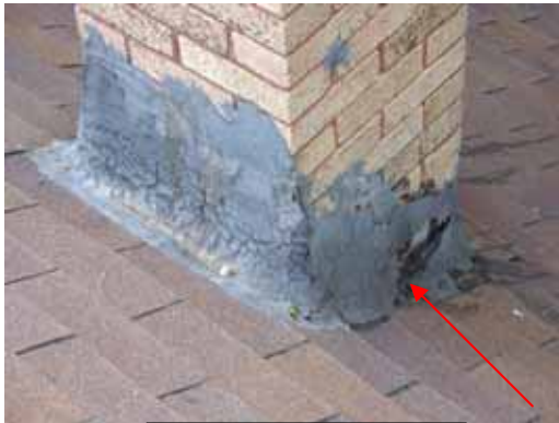
Not properly flashed
