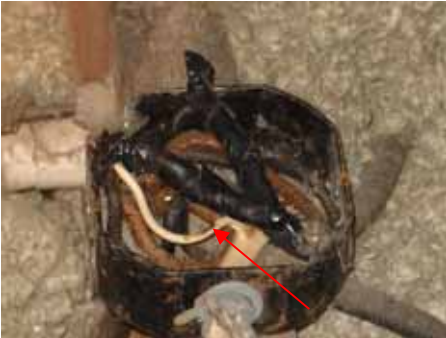
Missing cover and wire overheating
